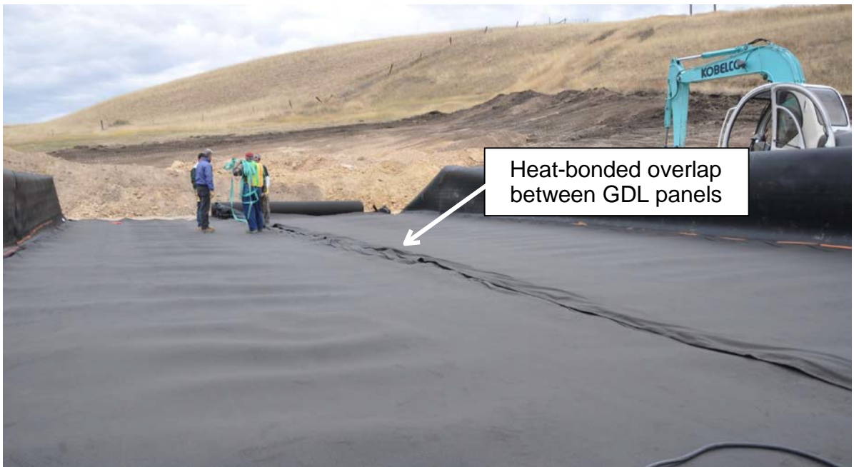
Figure 6. GDL being deployed on geomembrane (upper) and GDL fully deployed with heat-bonded overlap (lower). (Photos courtesy of Dr. Craig H. Benson)
