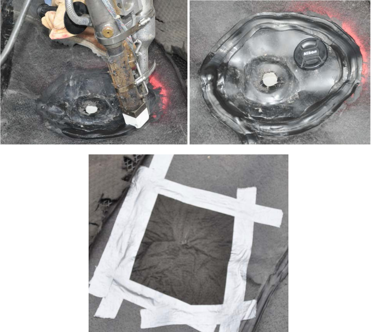
Figure 4. Welding geomembrane on base of lysimeter to percolation sump (upper left), completed weld and visible pipe for percolation (upper right), and non-woven geotextile secured over sump to prevent entry of debris into pipe (bottom). (Photos courtesy of Dr. Craig H. Benson)
