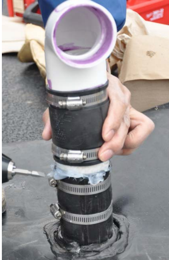
Figure 1. Rubber coupling used to ensure flexibility of boot for sump (Photo courtesy of Dr. Craig H. Benson)
