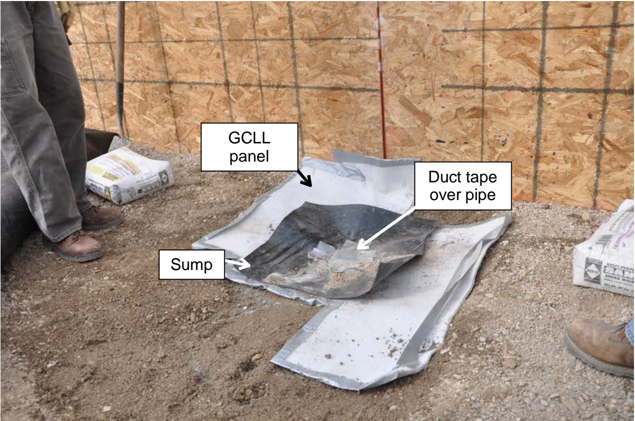
Figure 2. Sump installed on subgrade with duct tape sealing pipe opening and panel of GCL directly beneath sump. (Photo courtesy of Dr. Craig H. Benson)
